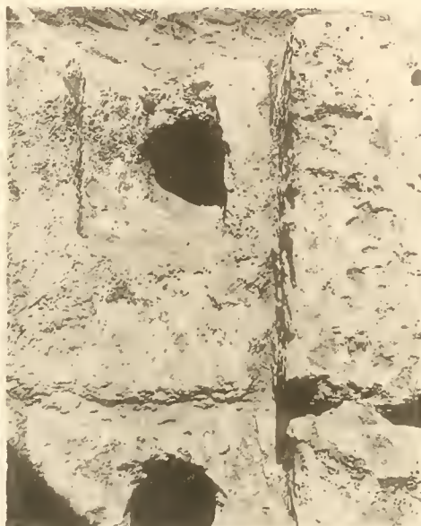
5. BOLT HOLES IN JAMB.
